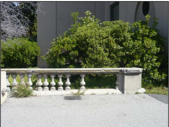
LOWER RIGHT: Short section of balustrade in obvious need of repair and replacement.
