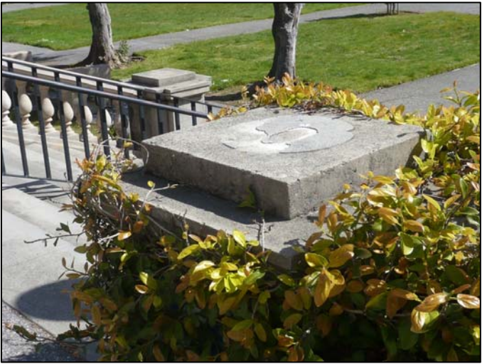
UPPER RIGHT: Pedestal of balustrade retains scars from missing spherical finial.
