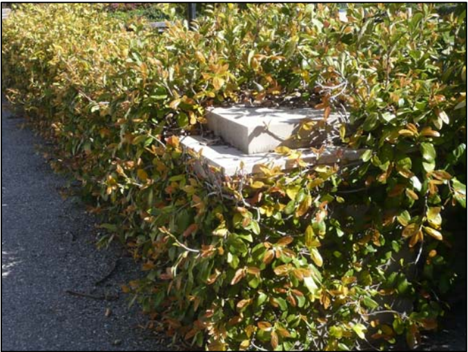
MIDDLE RIGHT: Pedestal of balustrade is barely visible due to overgrown plant material. Such growth must be removed with utmost care, under the direction and guidance of a materials conservator, to avoid damaging the historic material of the balustrade.
